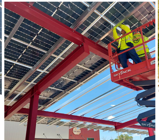
The solar carport outside the Zuni Major Market not only helps the market avoid electrical outages, but it also helps lower electricity costs. ©Alliance for Tribal Clean Energy
