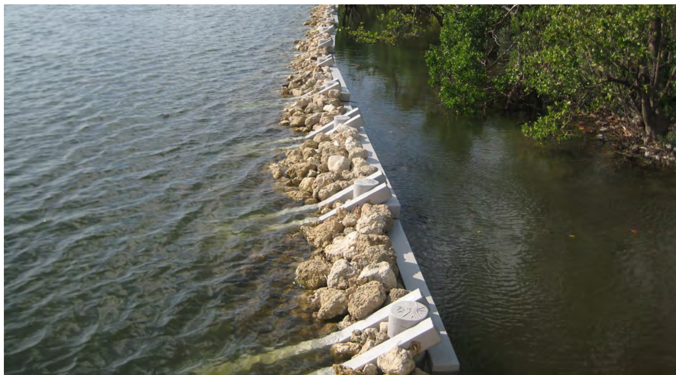
Riprap crib ©Paul Krashefski, Broward County EPCRD, 2011
