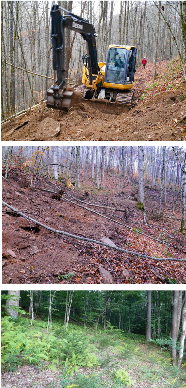
Fig. 8.14 A compacted logging road with minimal tree recruitment is being decomposed and outsloped with an excavator (top); newly decomposed and outsloped logging road within a northern hardwood forest provides an excellent opportunity for expanding red spruce coverage (middle); red spruce ( Picea rubens ) planted on the obliterated road a few years after treatment and planting (bottom; photos by Chad Landress)
