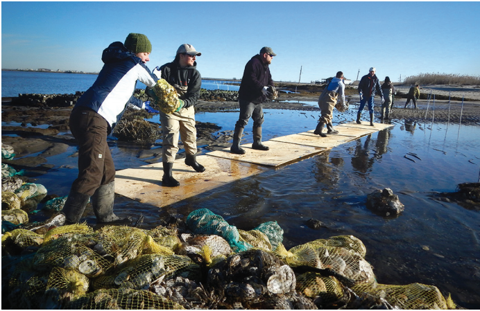
Volunteers, staff, and partners constructing a living shoreline with bagged oyster and clam shell. © The Nature Conservancy
