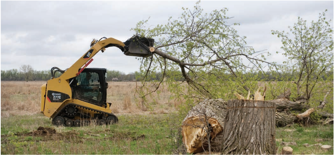
Skidsteer loader, piling trees that were cut to open up a prairie at the Conservancy's Central Platte River preserve in Nebraska. © The Nature Conservancy (Chris Helzer)
