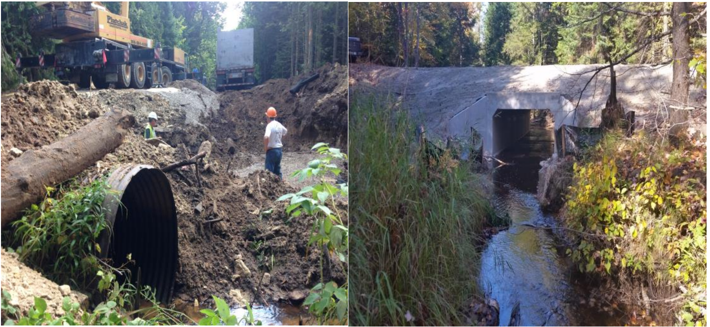
Before and After Images of the John's Creek Culvert. Photos Courtesy of The Nature Conservancy/Emily Clegg
