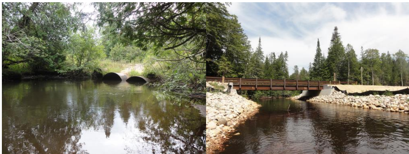
South Branch of the Two Hearted River road-crossing. Before: undersized culverts frequently overflowed, pulling sediment into the river. After: The new bridge has no affect on the natural flow of the river. Photo Courtesy of The Nature Conservancy/Emily Clegg
