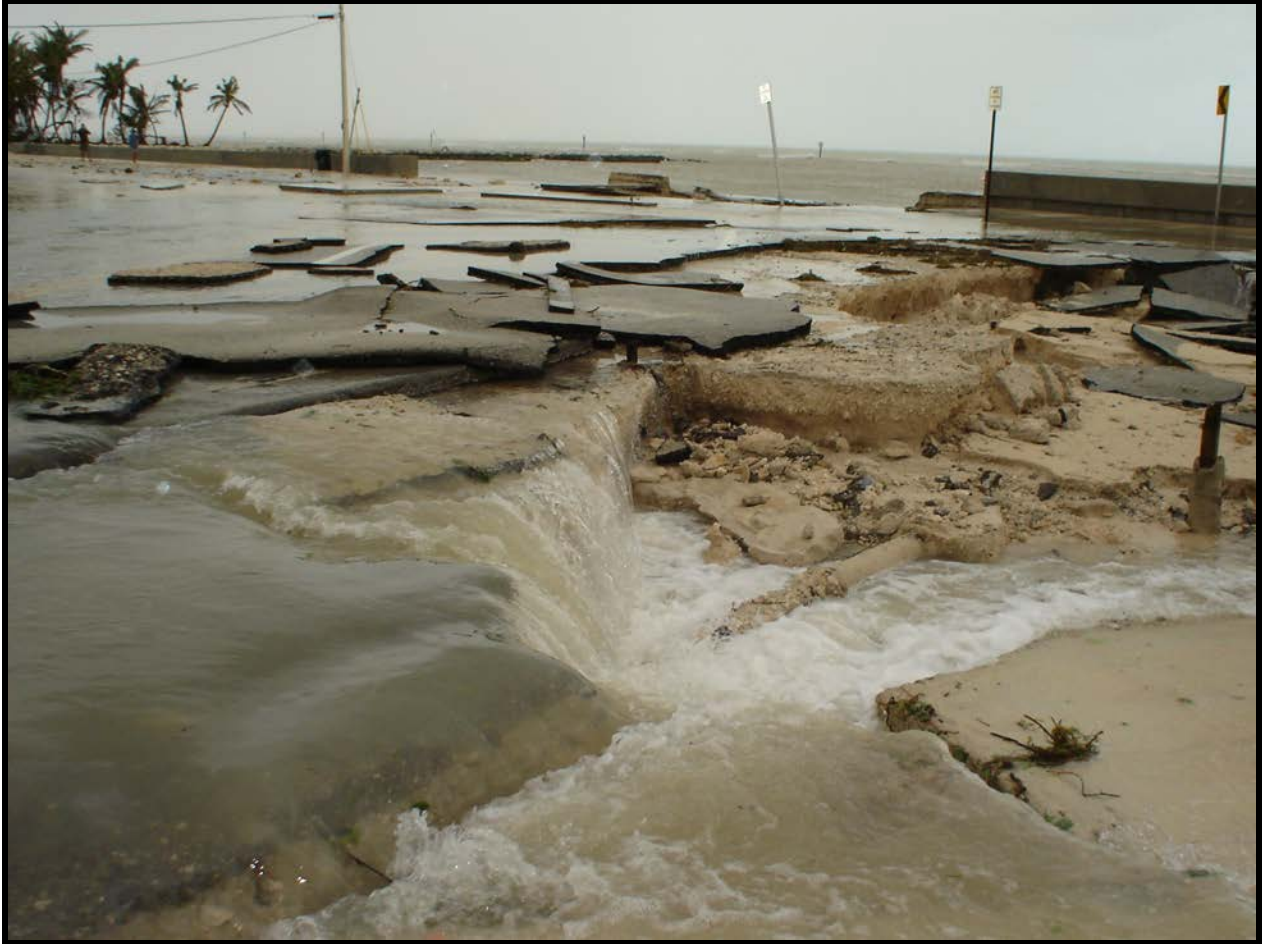
Fig. 11. Photograph of South Roosevelt Boulevard-Bertha Street intersection in Key West, FL around 1100 EDT, 24 October 2005. Note water flowing toward Hawk Channel (Atlantic Ocean) through large slabs of asphalt (photograph by Chip Kasper).
