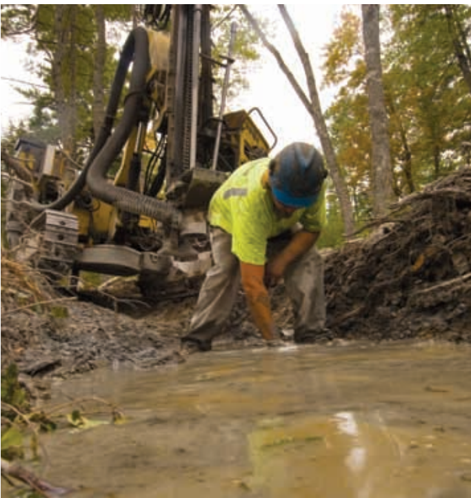
Using drilling equipment, workmen build a 17 step and pool waterway, which will allow thousands of alewife to access an adjoining stream for spawning. ©Bridget Besaw
