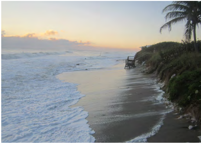
Dune Damaged by Hurricane Sandy, October 2012 ©Palm Beach County Environmental Resource Management
