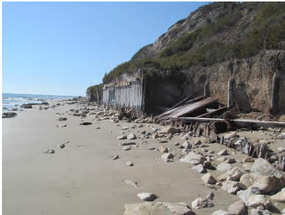
Photo 2-2. Condition of 1930s-Era Coastal Armoring along Goleta Coastline
