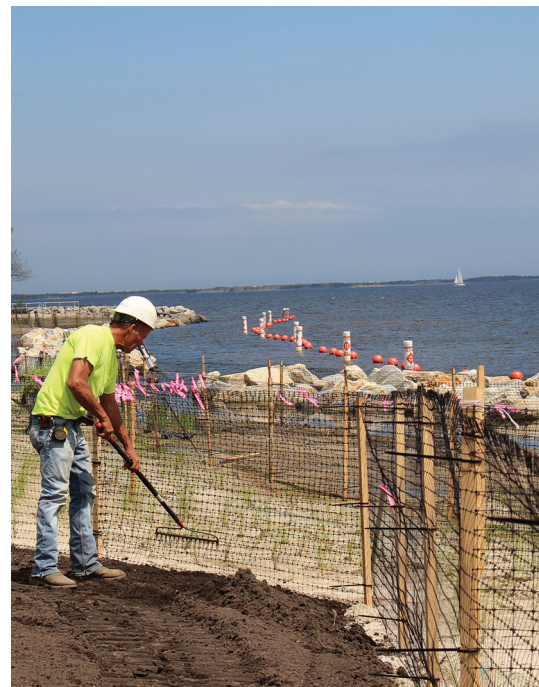
Upland planting behind rock sill living shoreline at Berkeley Island © T&M Associates
