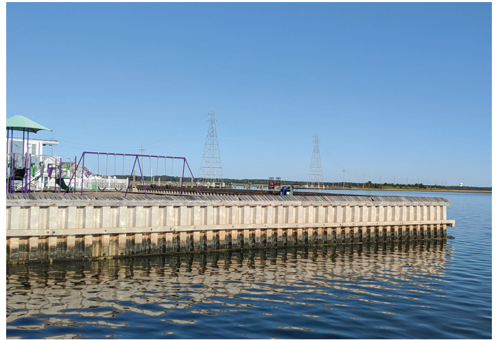
This vinyl bulkhead in Wildwood, NJ, is an example of a conventional gray shoreline stabilization project. © The Nature Conservancy
