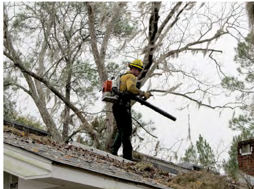
A Florida Forest Service ranger blows leaves from a roof as part of wildfire mitigation efforts.
