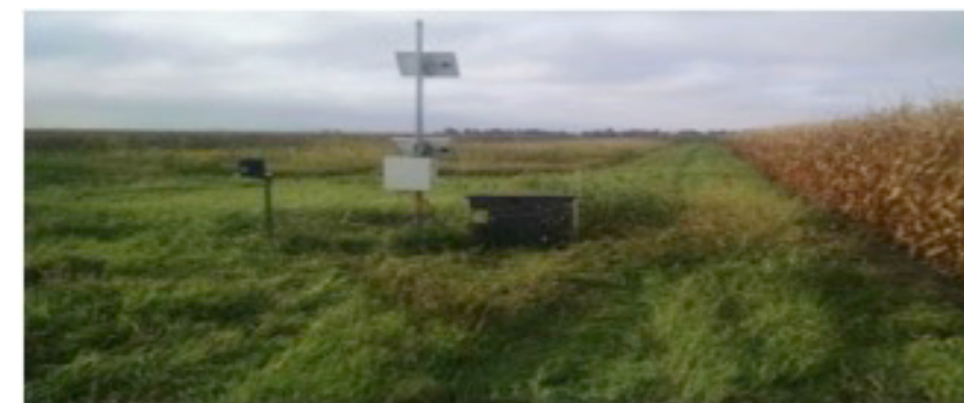
A control structure and monitoring equipment set up to monitor hydraulic conditions at a saturated buffer sight.
