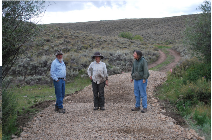
Completed low water crossing at West Fork, Wolf Creek on BLM lands
