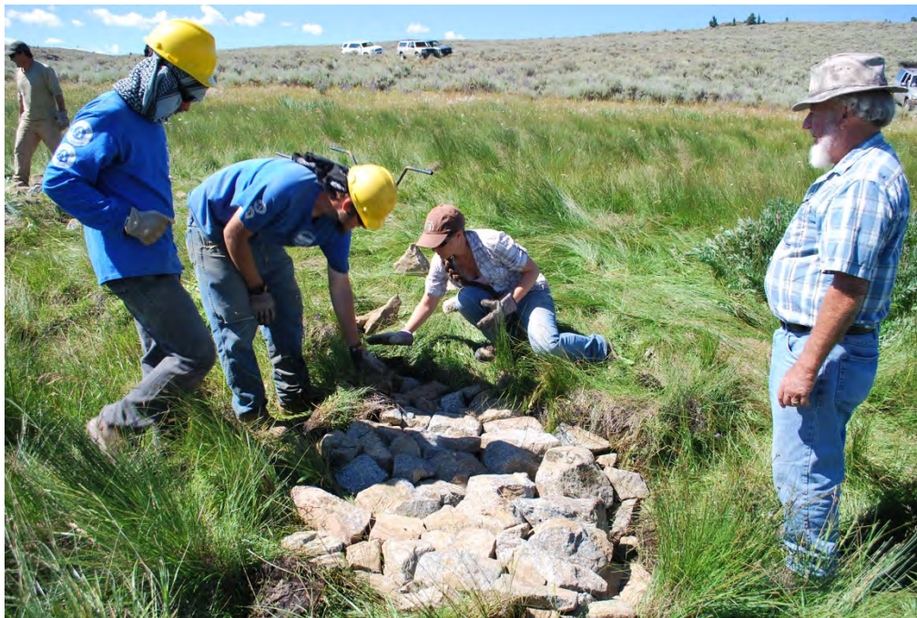
12. Hands-on training by Bill Zeedyk with Western Colorado Conservation Corps youth field crew members and Chayla Rowley, Natural Resources Conservation Service engineer, August 2014.
