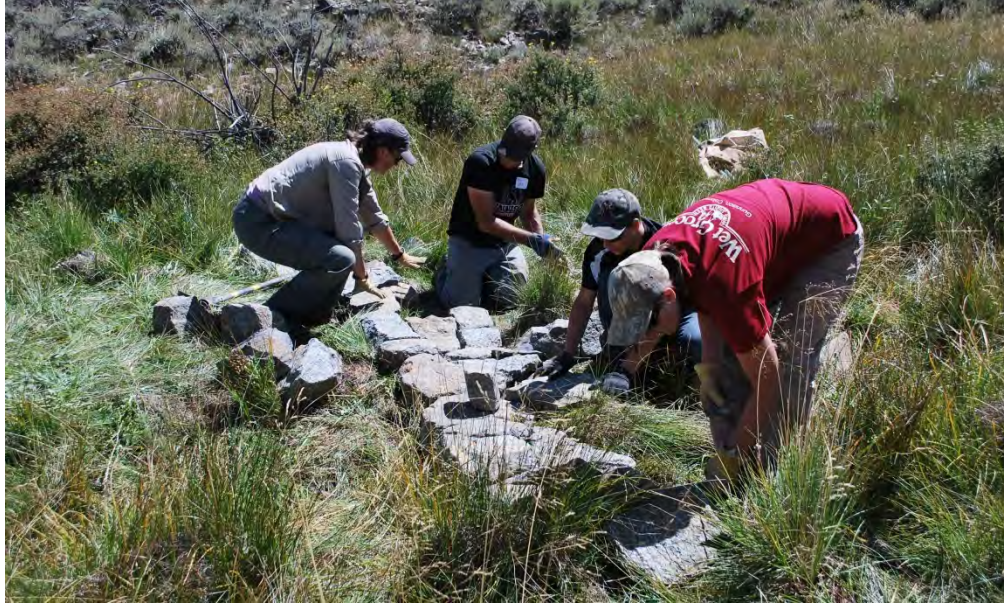
17. Gunnison High School Biology Class students and teachers build a one rock dam at Chance Gulch, Wildlands Restoration Volunteer event, September 2014.
