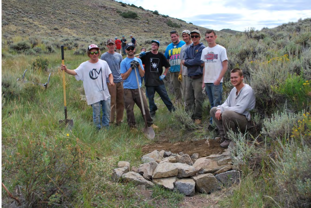
19. Western State Colorado University Ecological Monitoring class completes a one-rock dam in Chance Gulch, directed by Nathan Seward, Colorado Parks and Wildlife (in background), September 2014.
