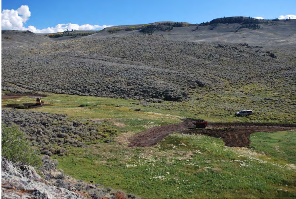
15. Stonefly Earthworks builds a “double bay plug and pond” structure at Moncrief Ranch, Kezar Basin, to rewet a meadow and reduce invasive species. NRCS planted native seed on the disturbed soil, September 2014.
