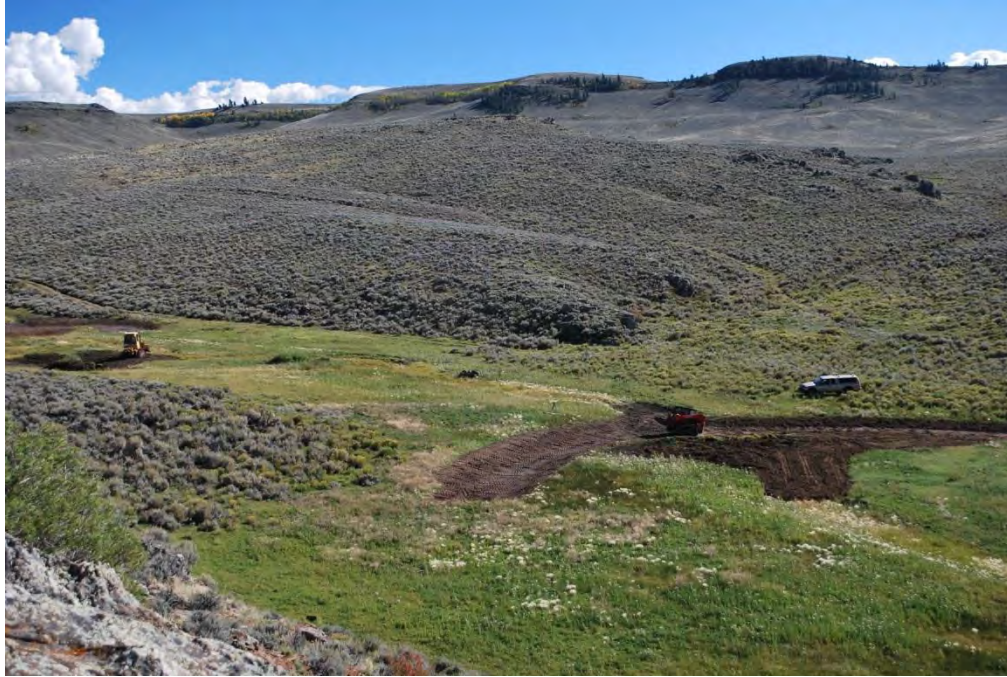
17. Stonefly Earthworks builds a “double bay plug and pond” structure at Moncrief Ranch, Kezar Basin, to rewet a meadow and reduce invasive species. NRCS planted native seed on the disturbed soil, September 2014.
