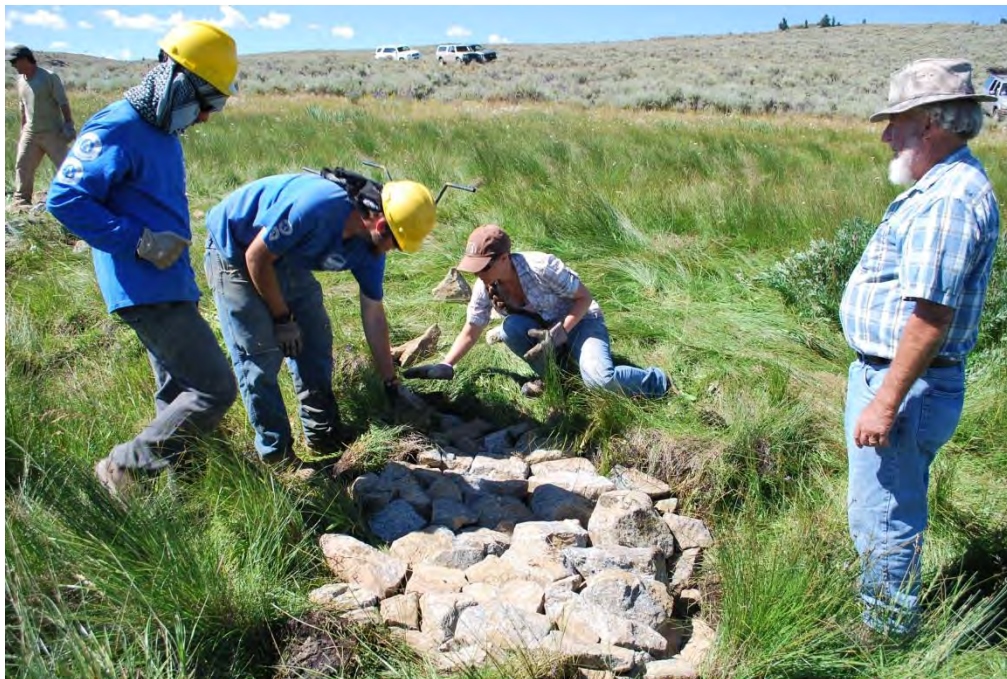
14. Hands-on training by Bill Zeedyk with Western Colorado Conservation Corps youth field crew members and Chayla Rowley, Natural Resources Conservation Service engineer, August 2014.
