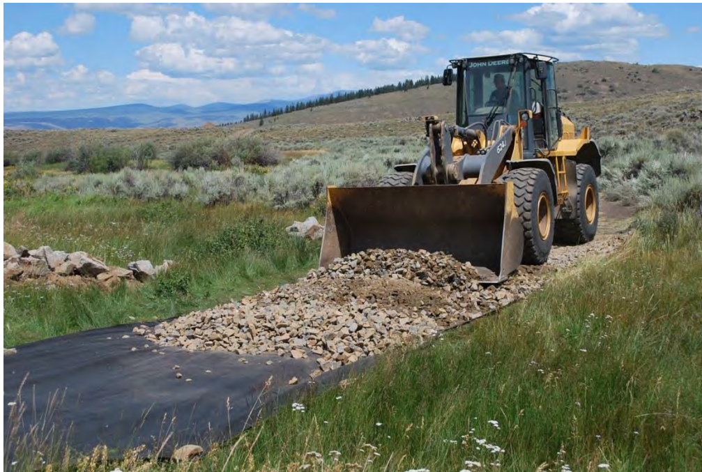
10. Gunnison Gravel front-end loader builds a low water crossing at Chance Gulch, August 2014.
