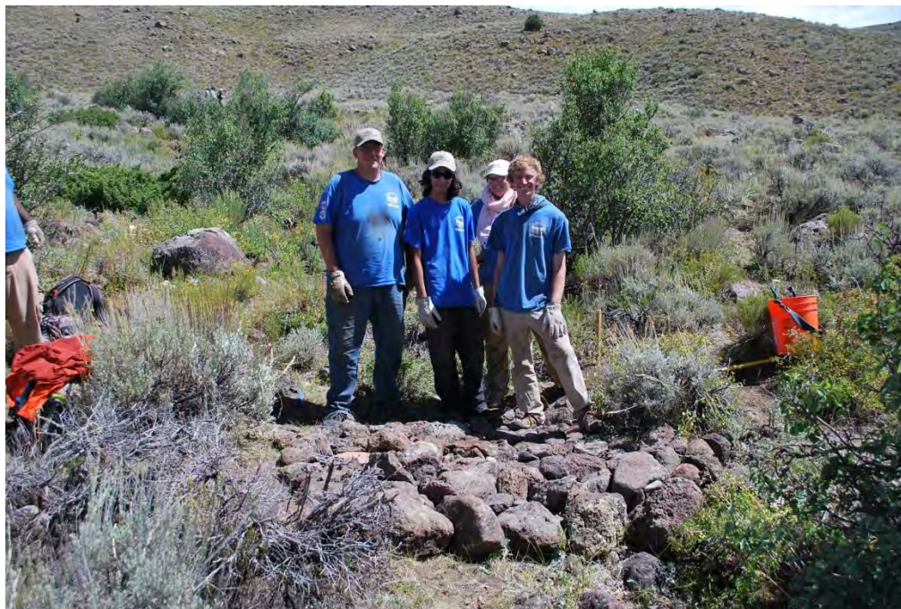
16. Western Colorado Conservation Corps field crew complete one rock dam structure at West Flat Top Mountain on US Forest Service lands above Redden Ranch, consisting of locally collected volcanic rock, August 2014.
