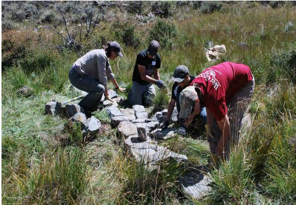
19. Gunnison High School Biology Class students and teachers build a one rock dam at Chance Gulch, Wildlands Restoration Volunteer event, September 2014.
