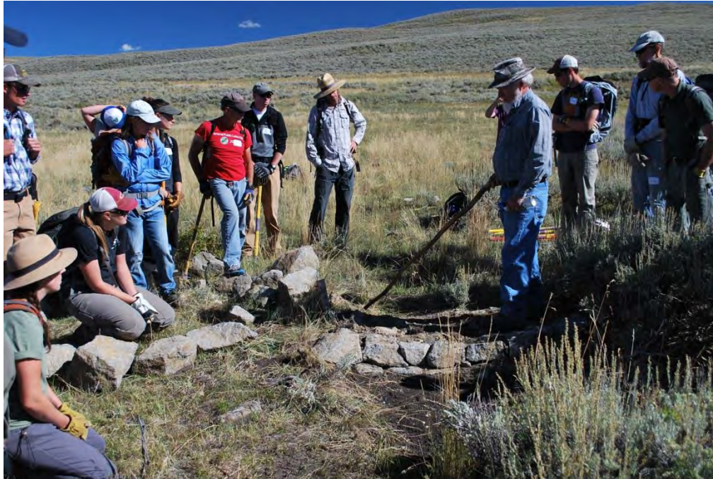
23. Bill Zeedyk explains the function of a one rock dam, a grade control structure, to volunteers and partners at West Flat Top Mountain during the Wildlands Restoration Volunteer five-day volunteer event, September 2014.
