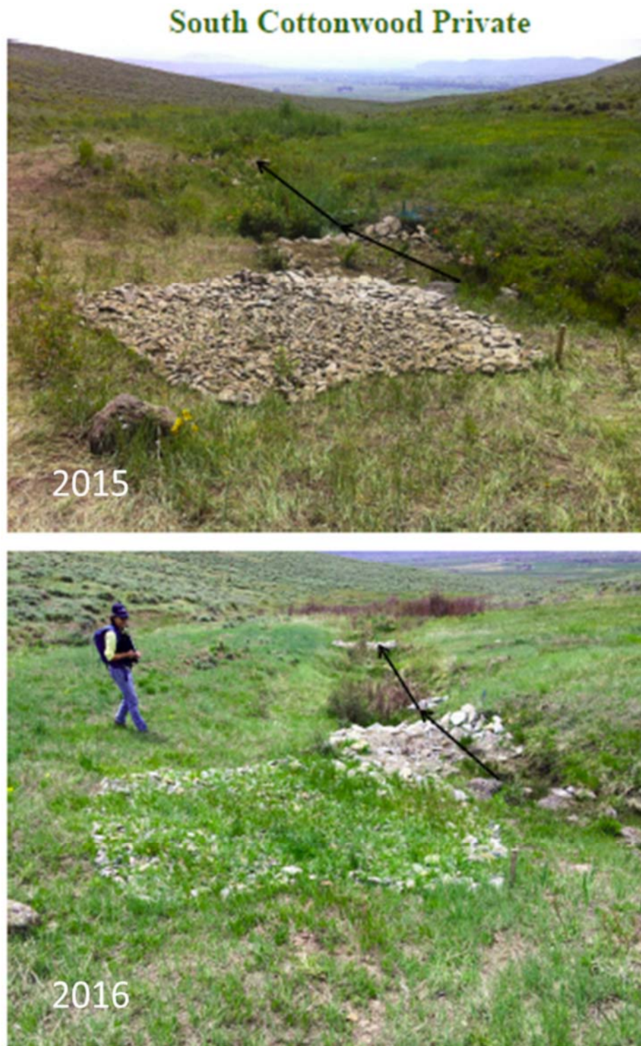
Top Photo: August 20, 2015 (structure completion date); Bottom Photo: May 26, 2016, Page 5 ➤ Arrows indicates direction of water flow and matches 2015 and 2016 photo positions
