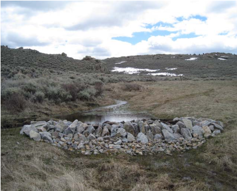
Figure 12. Filter dam at Chance Gulch (top) and one rock dam at Chance Gulch (bottom). Both photos by Andrew Breibart, BLM.
