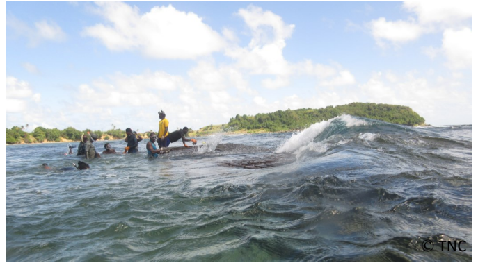
Building the reef breakwater, one stone at a time. Packing the second layer of baskets at low tide with waves now breaking directly on the breakwater.
