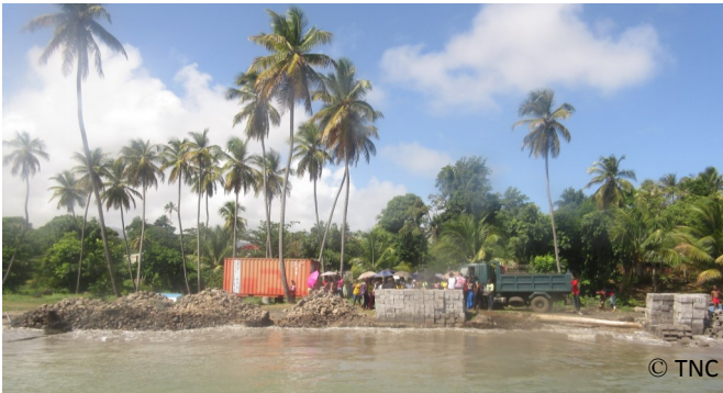
Telescope Beach - Grenada. The mobilization site for the Reef Engineering and Restoration Project where all materials and equipment were kept during construction. The site was landscaped on completion
