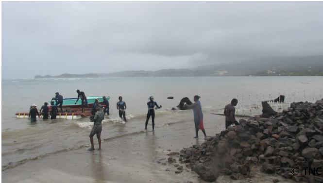
Loading the barge with rocks from the beach, done manually by a team of 10 spearfish divers from the Grenville community.
